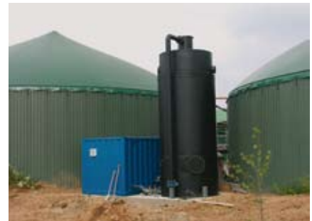
Desulfurization of biogas
