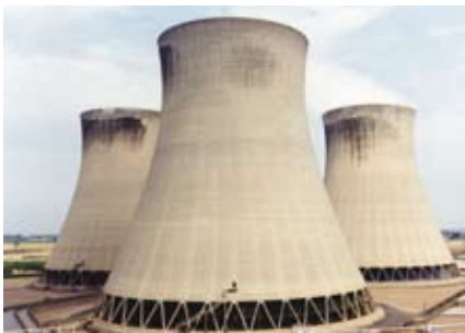
2H- PLASdek® DRAX, Great Britain: Replacement and upgrade of fills (1999, 2001)
