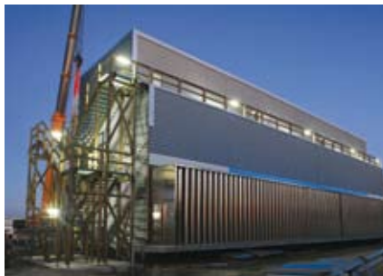
2H- PLASdek® Unterhaching, Germany: First installation of fills and drift eliminators (2006)
